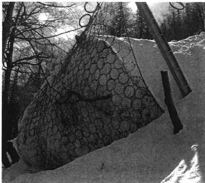
Figure 10 – Flexible Avalanche Barrier Photo
